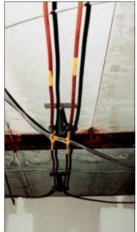
A clever bracket system made installation of the copper tube easier in the corridors.
