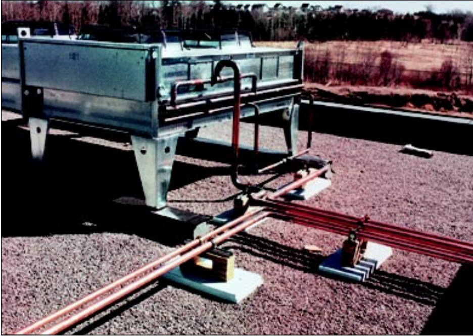
The roof mounted fan coil heat exchangers are connected to the refrigeration system by runs of copper tube.
