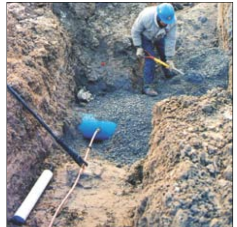
Backfilling of an underground water installation, showing the main, service, anode and curb stop.
