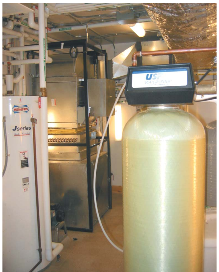
Copper was a key component in the design and installation of the water and cooling systems.
