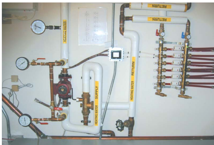
A copper-intensive control panel for some of the mechanical systems in the Inn.
